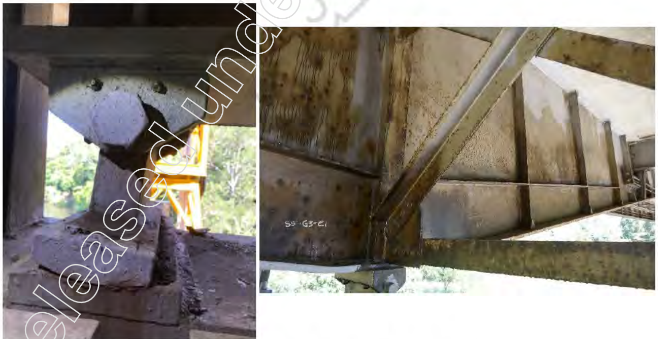
Figure 42: Existing rocker bearings on bridge and corrosion on the steelwork
