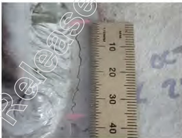
Figure 19: Crack at weld toe/HAZ, Cross Girder 3 flange to Web G1.
