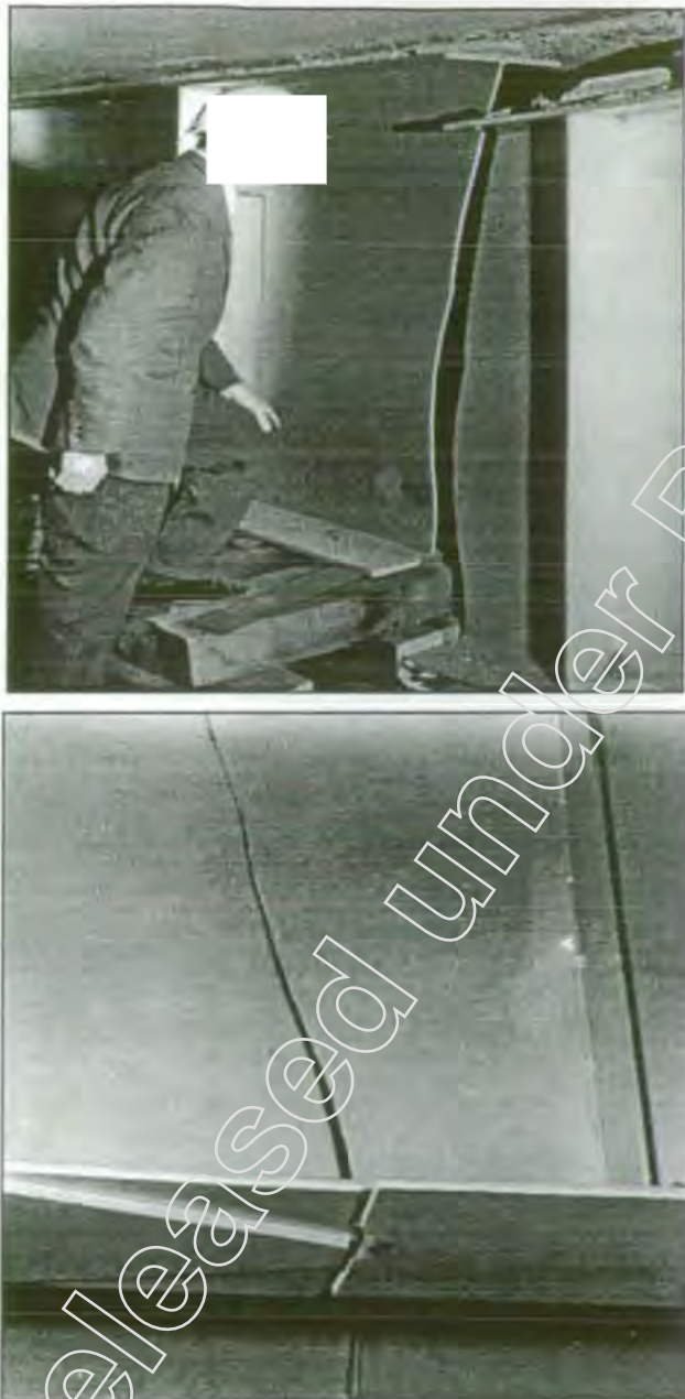
Figure 3: Example of brittle fracture at Kings Bridge Melbourne.
