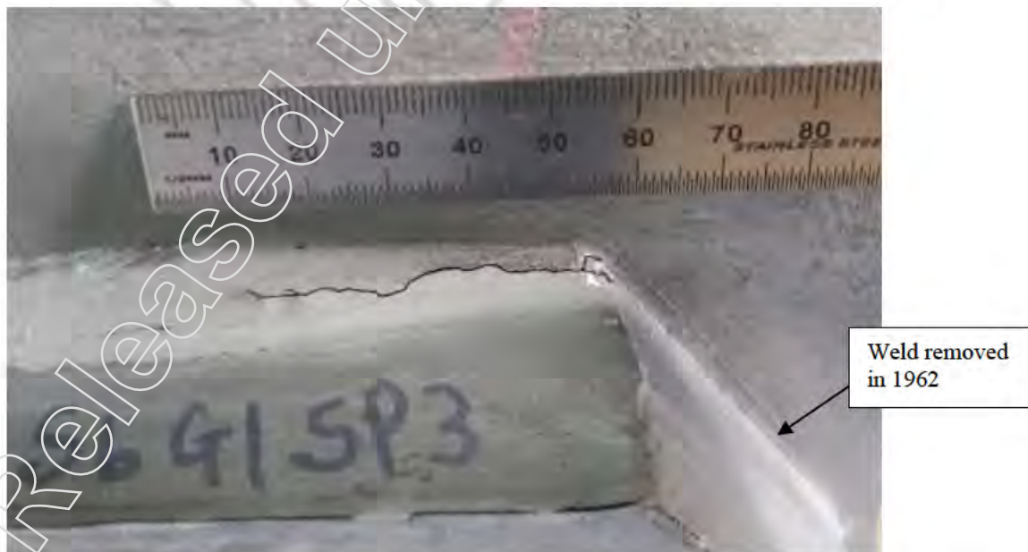
Figure 4: 53mm crack in span 6 edge girder. Note end fillet weld removed during 1962 strengthening
