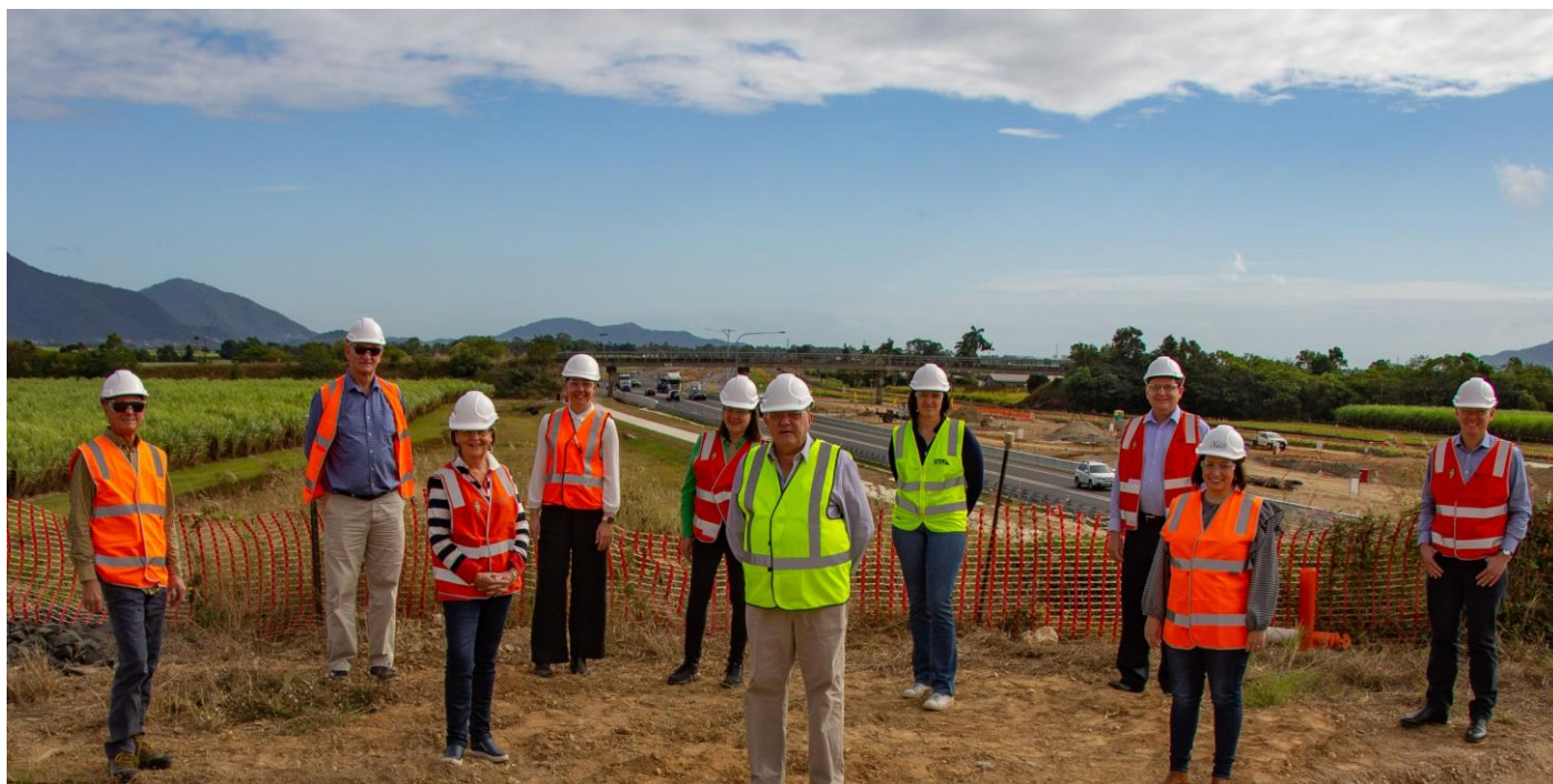
BHTAC members at the site for the new overpass at Maitland Road (Bruce Highway in background). This location is within the footprint of the Cairns Southern Access Corridor (Stage 3), Edmonton to Gordonvale project, currently under construction.
