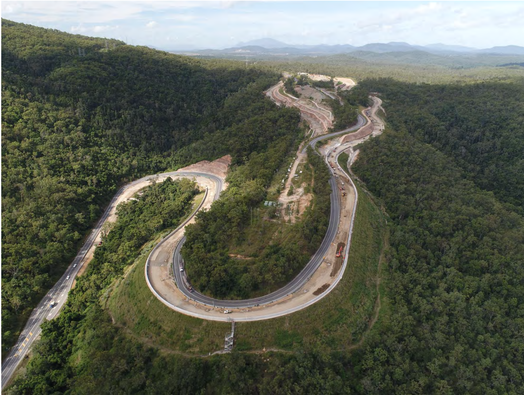
Figure 3: View of the Project, looking from the north. The upcoming traffic switches will move the Peak Downs Highway traffic onto the northbound (outer) carriageway.
