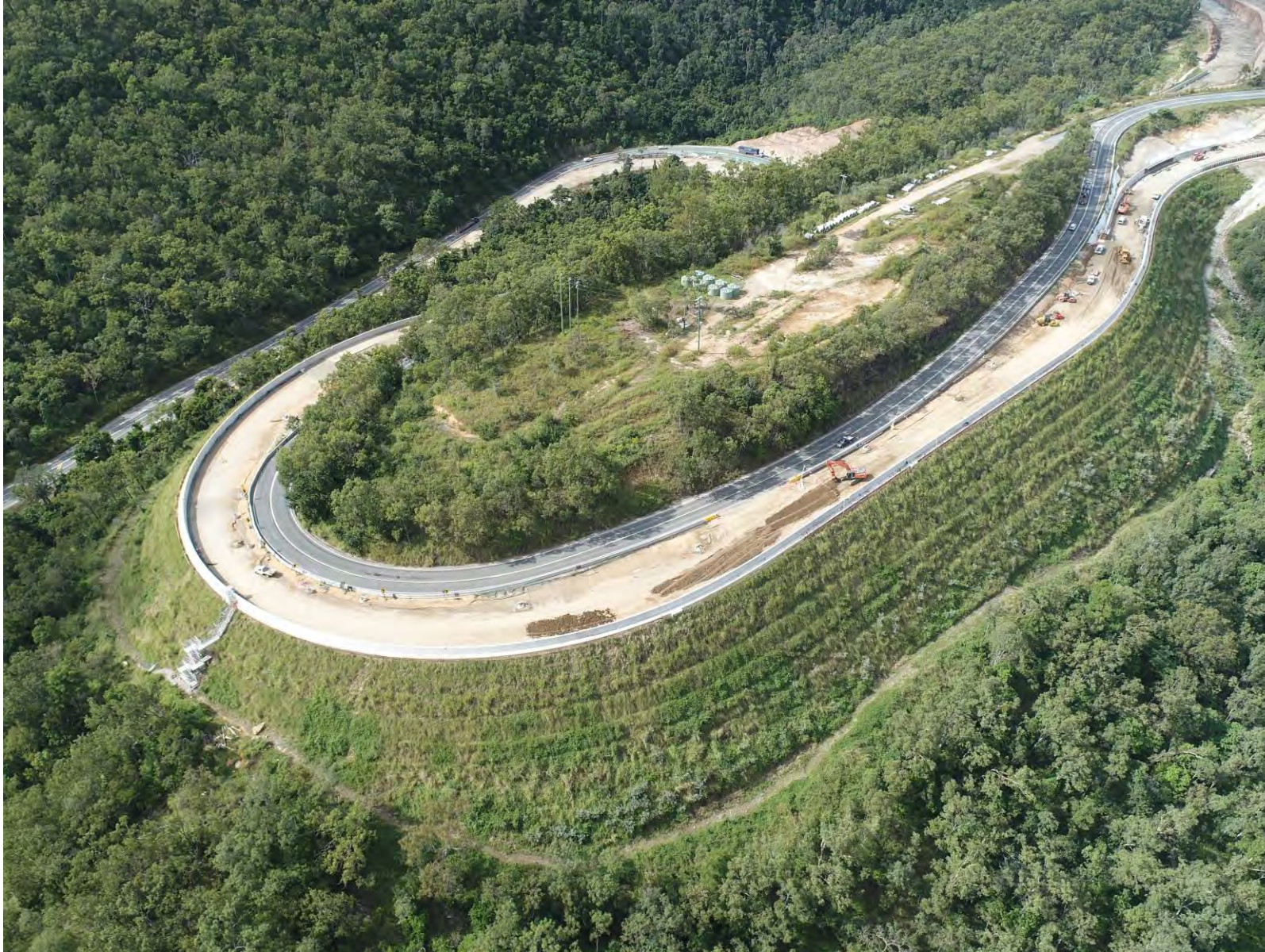
Figure 2: The Project's major Reinforced Earth Embankment (REE) is now complete and landscaped
