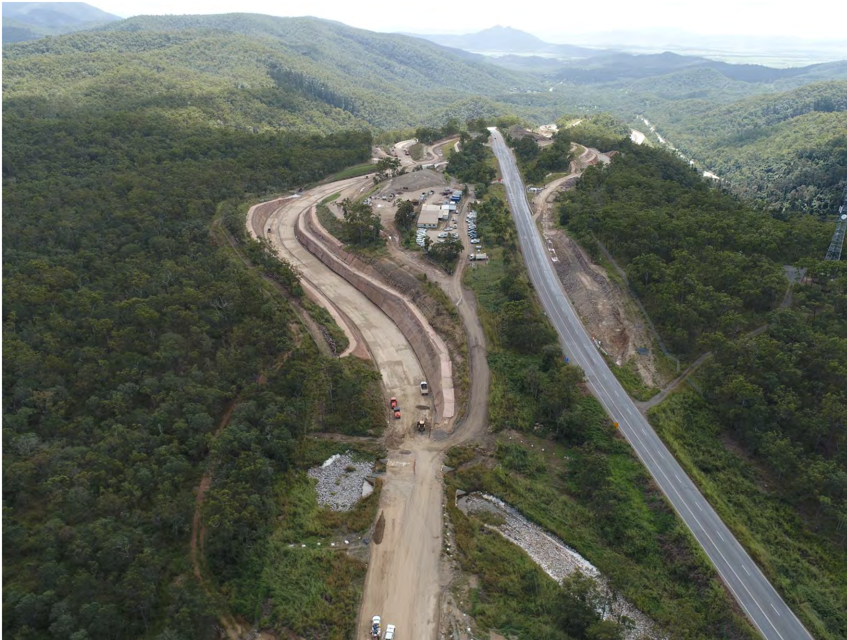
Figure 4: View from the south with the existing Peak Downs Highway right of picture and the new northbound alignment left of picture
