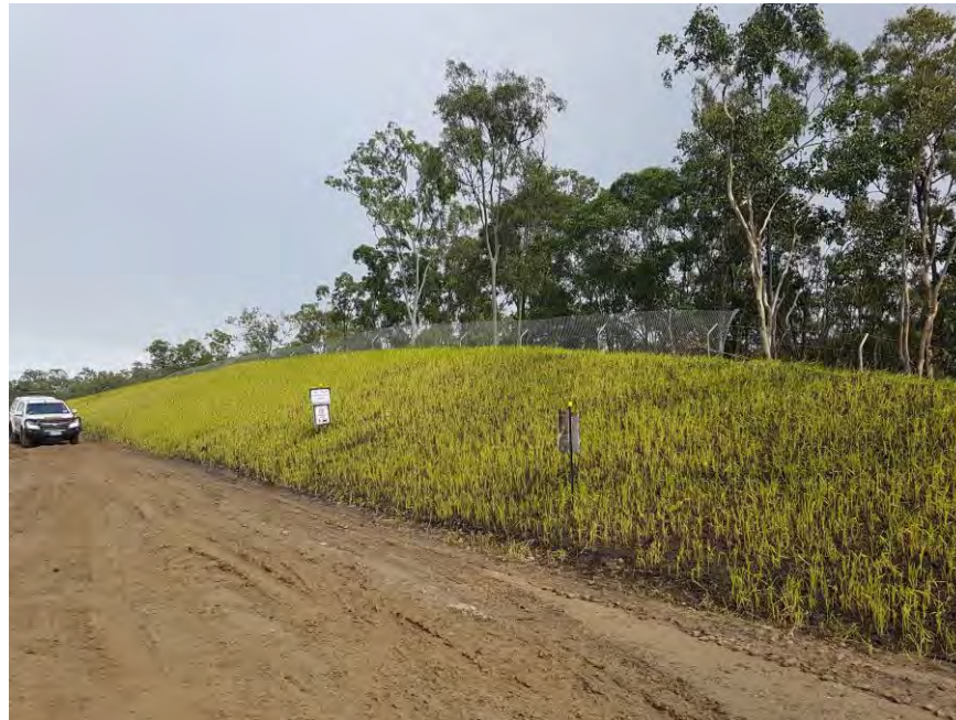
Figure 11: Recent organic blanket treatment on a road cut adjacent to fauna exclusion fencing under construction.
