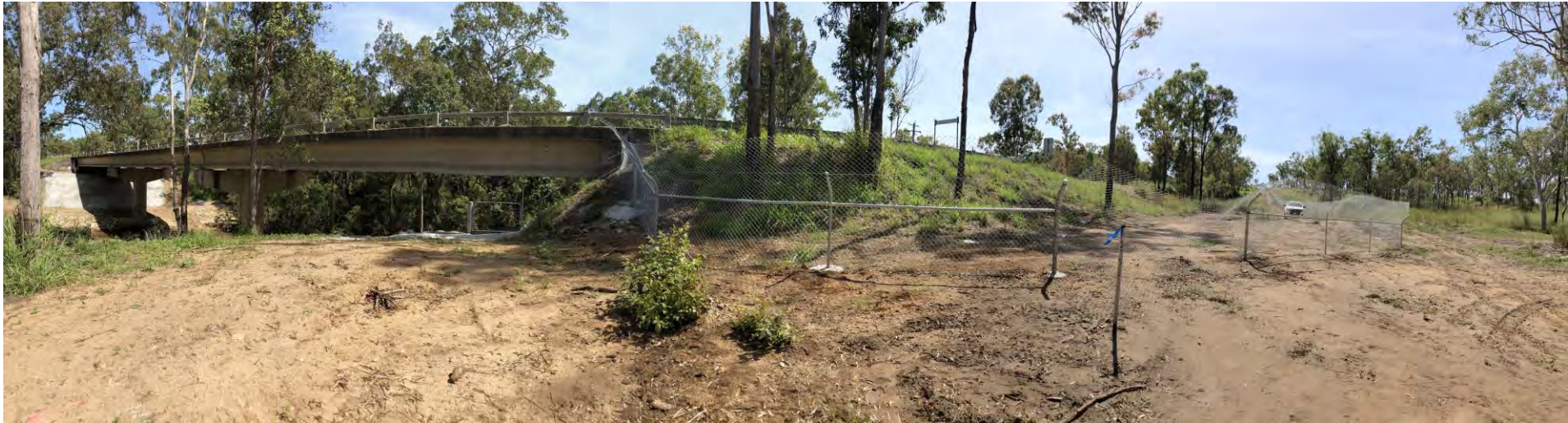
Figure 14: Fauna exclusion fencing erected adjacent to Denison Creek in April 2019, directing animals to pass underneath the bridge
