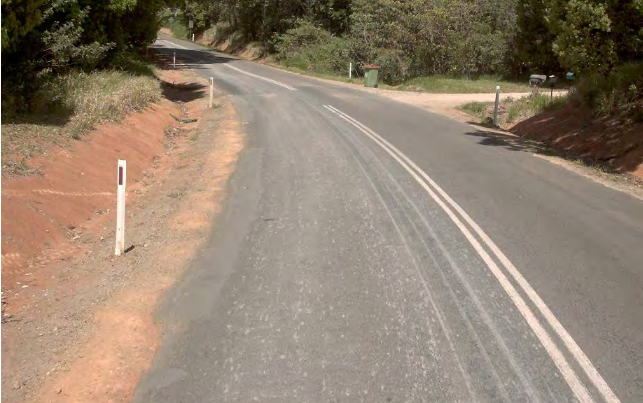
Figure 17 - Photo showing that vehicles utilise the gravel/unsealed shoulders
